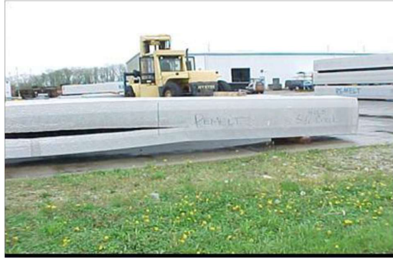
Unsafe Crack for Ingot
